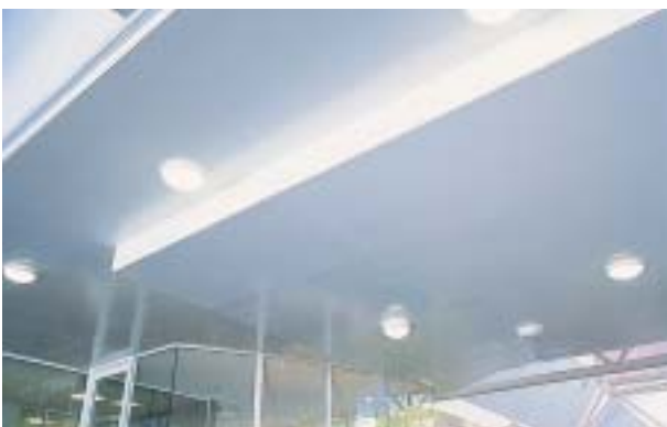
Duralux™ fibre cement sheets to ceiling and bulkheads adjoining the administration centre.
