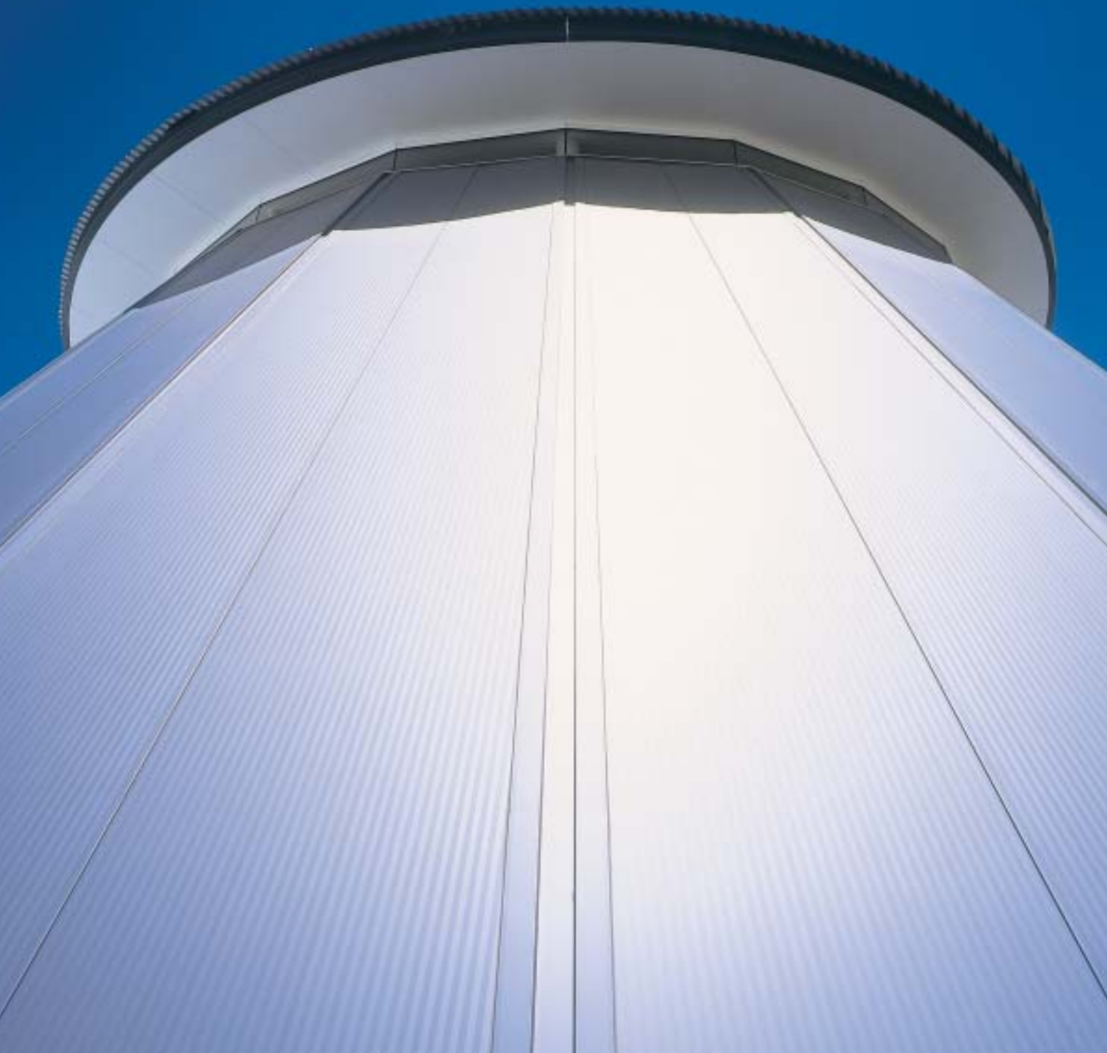
Soffit lining to the 'Cone Dome' of the childrens play gym comprises 6.0mm BGC Duralux™ fibre cement sheets.
