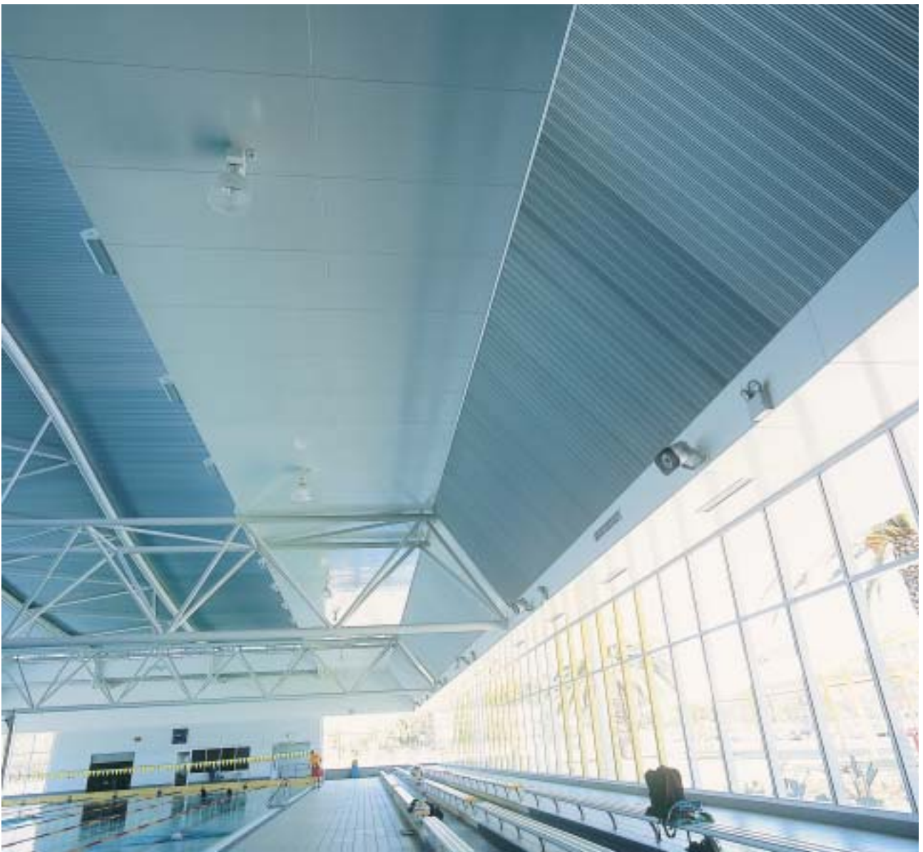
Ceiling treatment to the main pool comprises 6.0mm BGC Duralux™ fibre cement sheets
